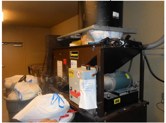
Chute was full because compactor was.
